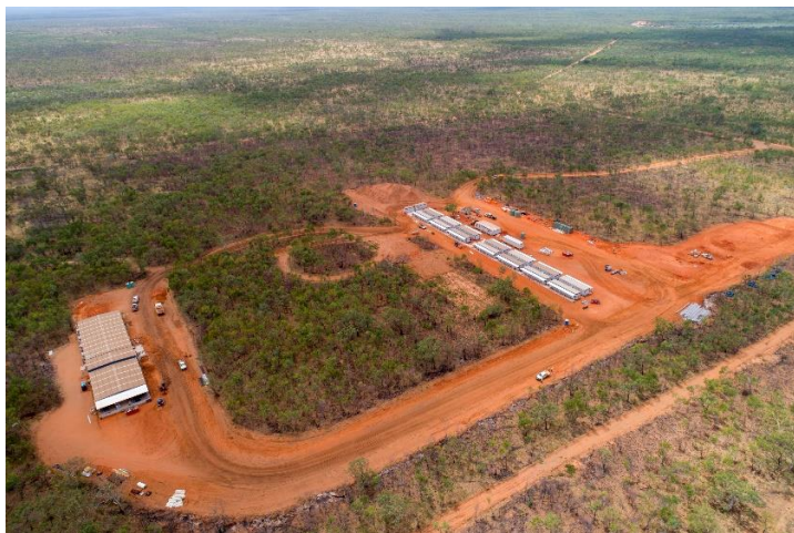
Taking shape on site - the Village to house the Thunderbird construction workforce.
